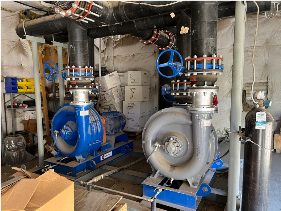
Picture 2: Blowers for Gas Flare Inside Shed
