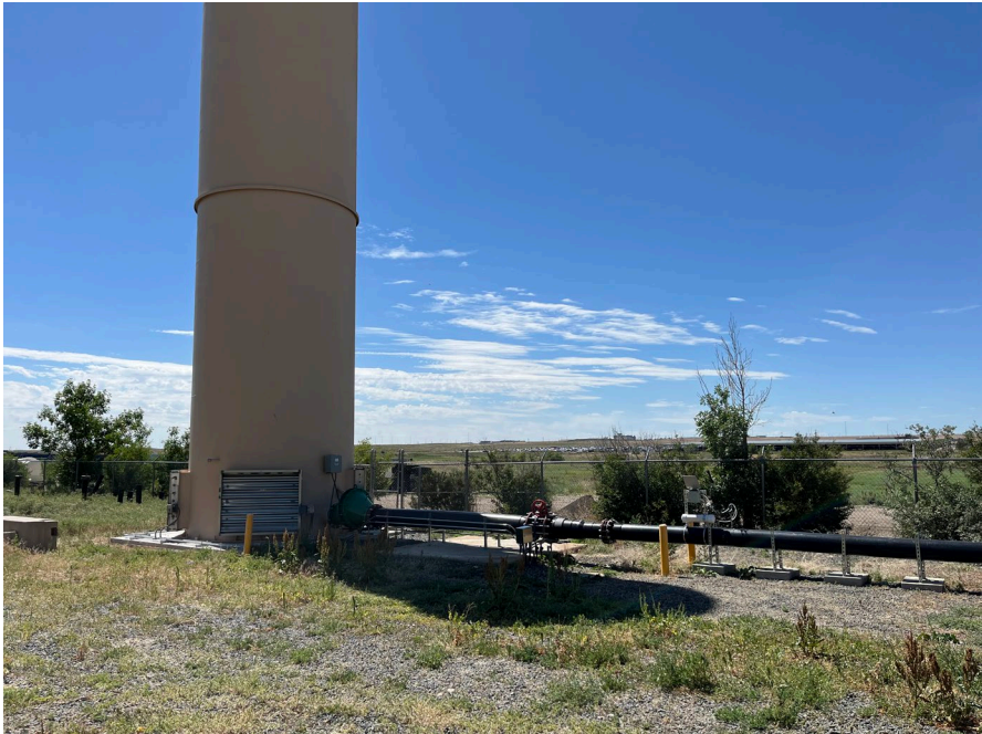
Picture 1: Gas Flare Looking Southeast
