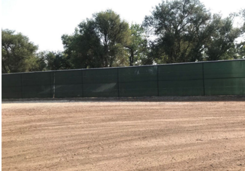
Photos of the 25 foot demarcation pole and 8 foot screen wall on site
