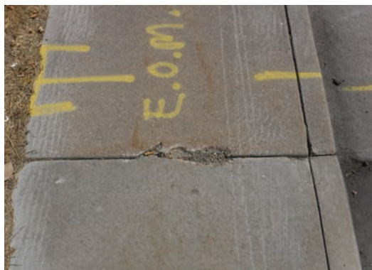
Cracked/Uneven Pedestrian Surfaces
