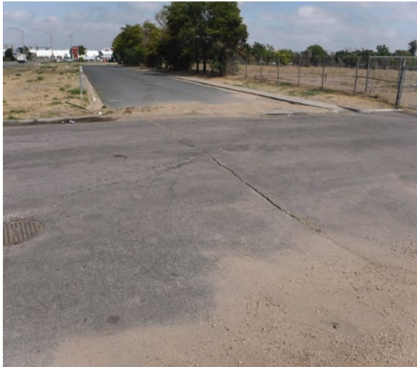
Lack of Access to Dahlia Street right-of-way
