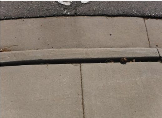
Cracked/Uneven Pedestrian Surfaces
