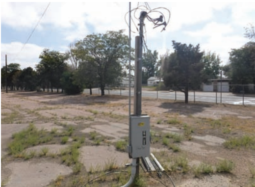
Deteriorated Electrical Pole
