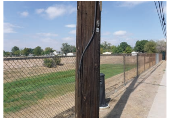
Unsafe/Exposed Electrical Wire
