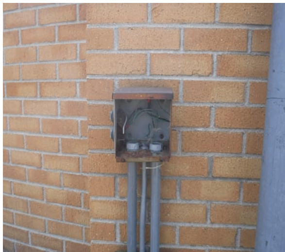
Unsafe/Exposed Electrical Wire
