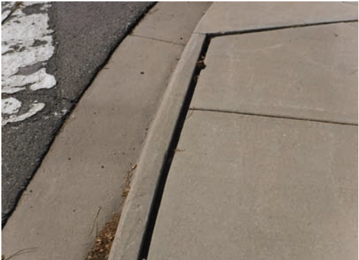
Cracked/Uneven Pedestrian Surfaces
