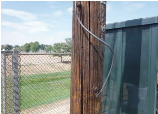
Unsafe/Exposed Electrical Wire
