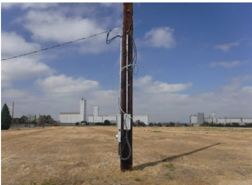
Deteriorated Electrical Pole
