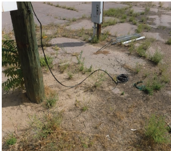
Unsafe/Exposed Electrical Wire
