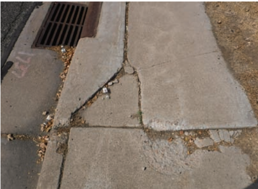
Cracked/Uneven Pedestrian Surfaces
