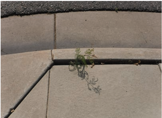
Cracked/Uneven Pedestrian Surfaces
