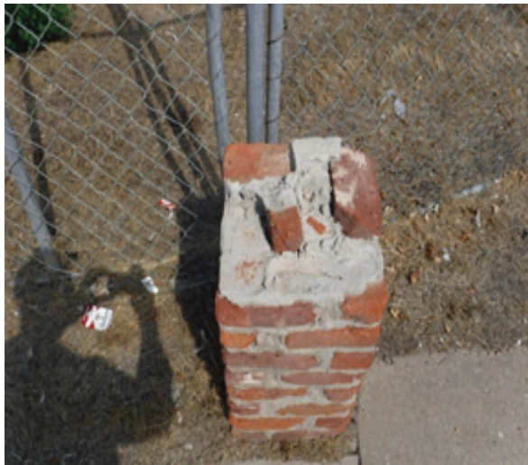
Deteriorated Support Post
