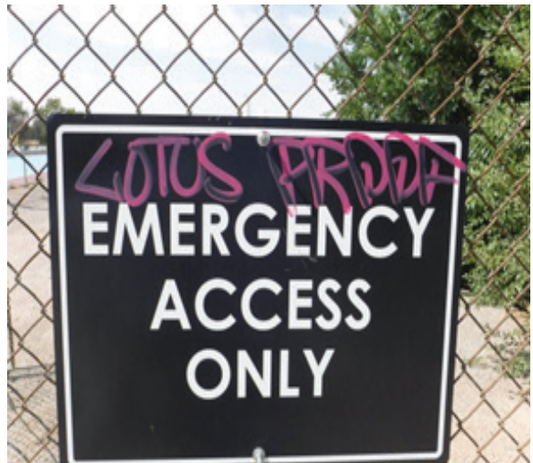
Deteriorated Signage via Graffiti
