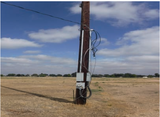
Deteriorated Electrical Pole
