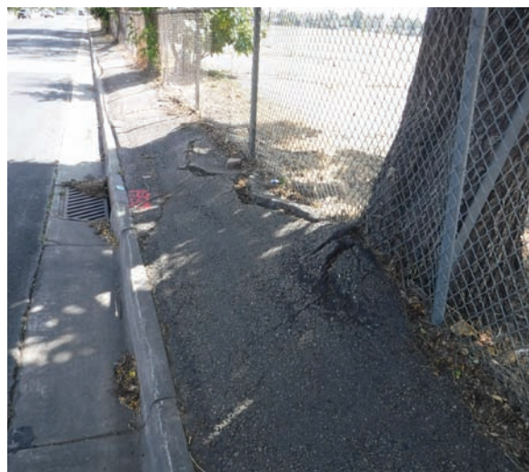
Lack of Sidewalk
