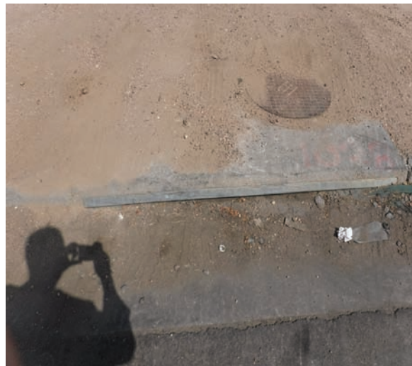
Deteriorated Stormwater Systems
