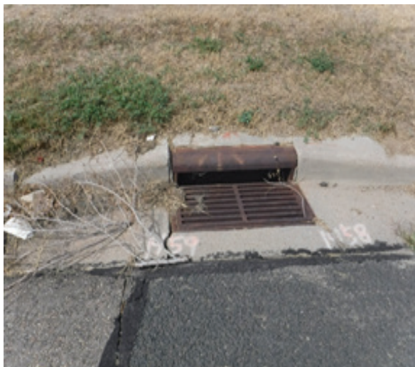
Deteriorated Stormwater Systems
