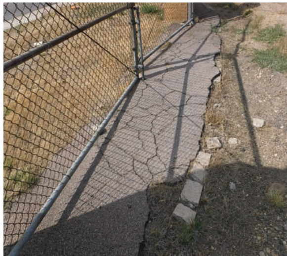
Blocked/Poorly Maintained Emergency Access
