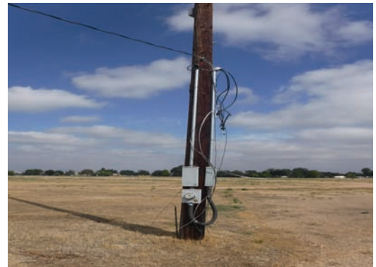
Deteriorated Electrical Pole
