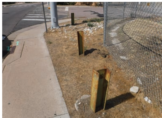
Deteriorated Accessory Structure
