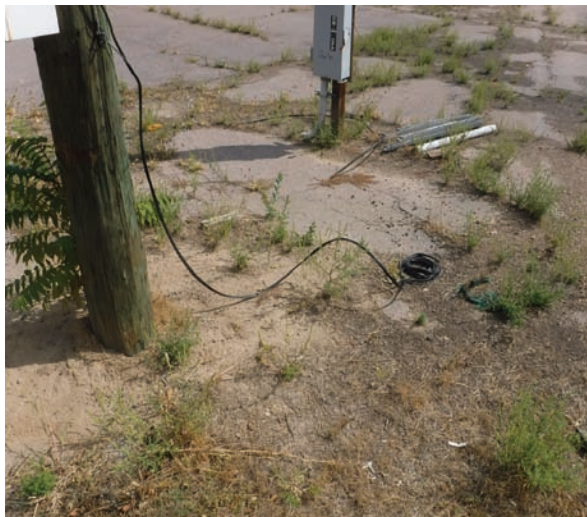
Unsafe/Exposed Electrical Wire
