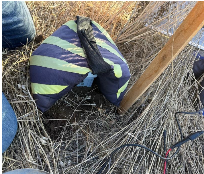
Photo 1: Installed Vibration Monitor
