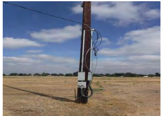
Deteriorated Electrical Pole
