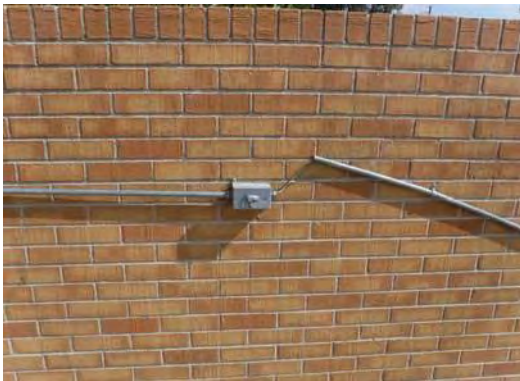
Unsafe/Exposed Electrical Wire
