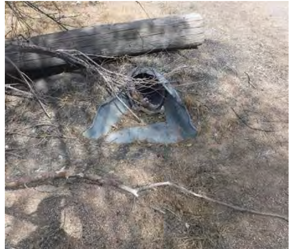
Deteriorated Stormwater Improvements
