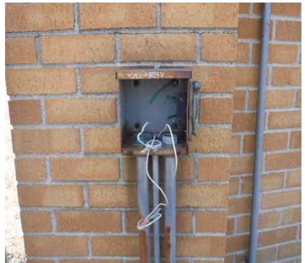
Unsafe/Exposed Electrical Wire
