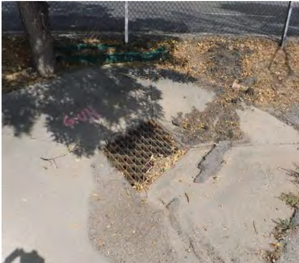
Deteriorated Stormwater Improvements
