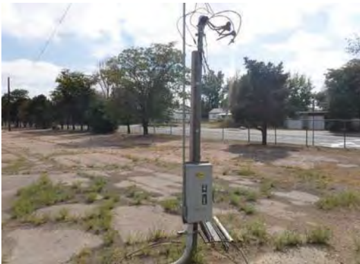
Deteriorated Electrical Pole
