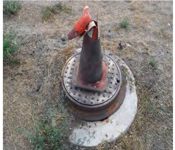
Dilapidated/Deteriorated Accessory Structure
