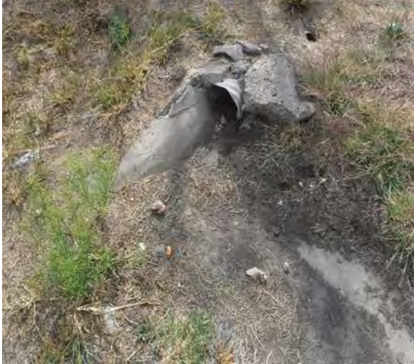
Deteriorated Stormwater Improvements
