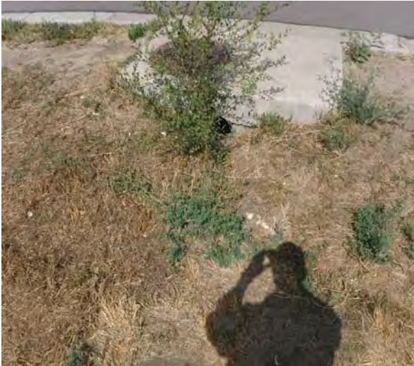
Deteriorated Stormwater Improvements
