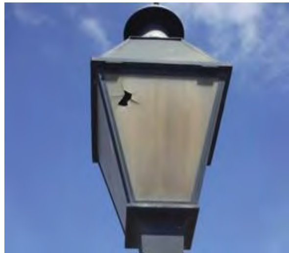
Deteriorated Light Structure
