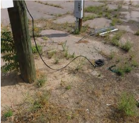
Unsafe/Exposed Electrical Wire
