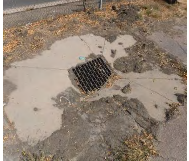
Deteriorated Stormwater Improvements
