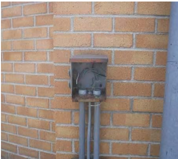
Unsafe/Exposed Electrical Wire
