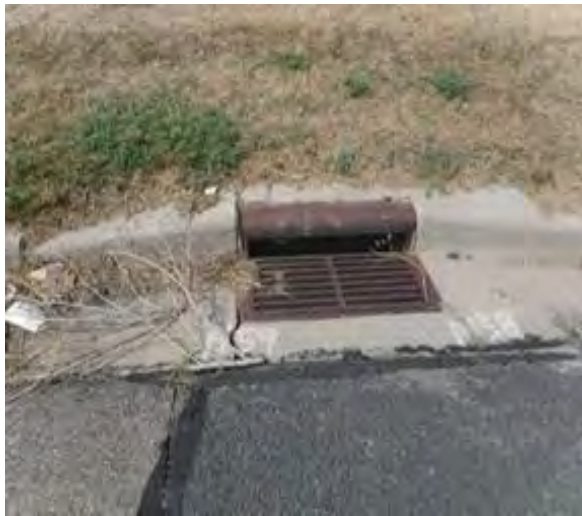
Deteriorated Stormwater Systems
