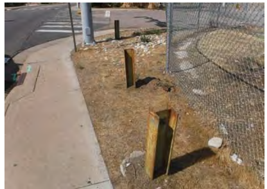
Deteriorated Accessory Structure
