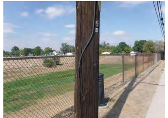
Unsafe/Exposed Electrical Wire
