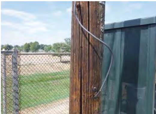
Unsafe/Exposed Electrical Wire
