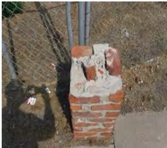
Deteriorated Support Post
