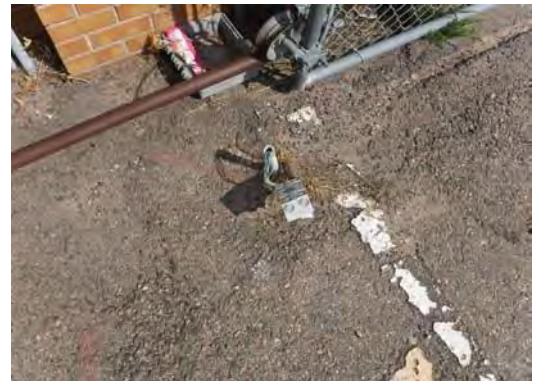
Unsafe/Exposed Electrical Wire
