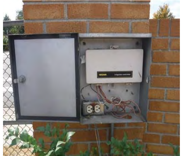
Unsafe/Exposed Electrical Wire
