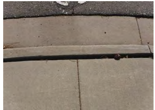
Cracked/Uneven Pedestrian Surfaces
