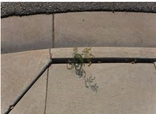
Cracked/Uneven Pedestrian Surfaces
