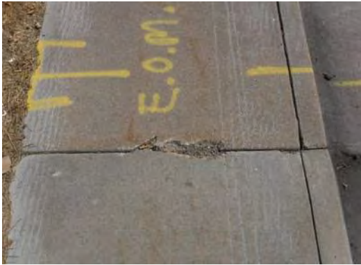
Cracked/Uneven Pedestrian Surfaces
