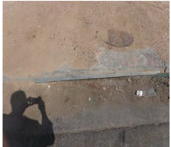
Deteriorated Stormwater Systems
