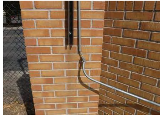
Unsafe/Exposed Electrical Wire
