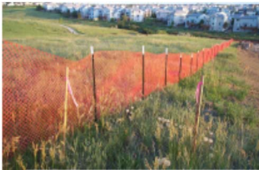
Use construction fence to restrict access to site and demark limits of disturbance.
