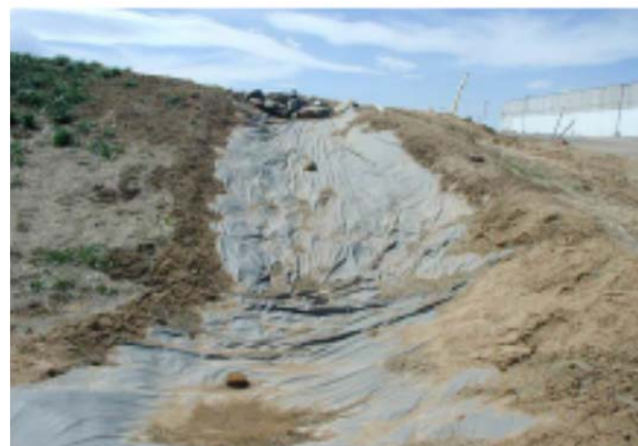
This plastic lined temporary slope drain allows runoff to be conveyed down a slope without causing rill and gully erosion.
