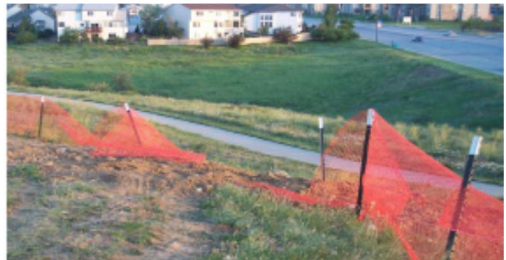
This construction fence is in need of repair. Inspections shall be made weekly and downed sections repaired immediately.
