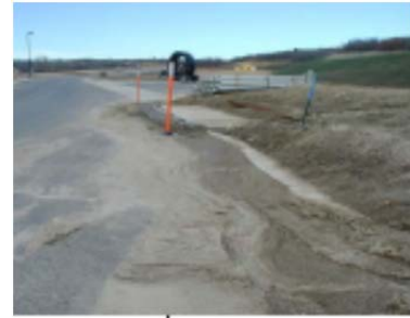
This inlet protection is overdue for sediment removal.
