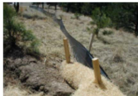
Silt fence is to be securely tied into adjacent BMP's such as the sediment control log shown here, or reinforced rock berms or sediment basin embankments.
