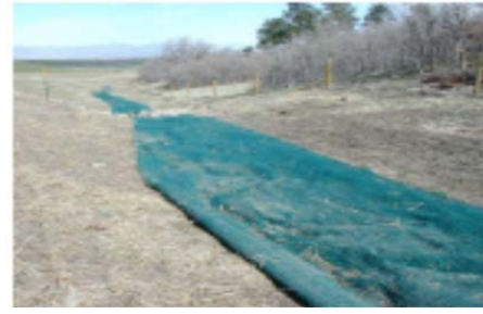
The edges of this erosion control blanket are not trenched in, allowing the blanket to become displaced. Blanket shall be 100% natural and biodegradable.
