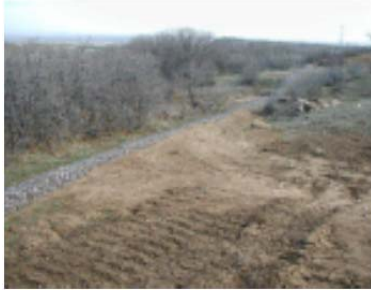
A reinforced rock berm may be used downgradient of disturbed areas in lieu of silt fence.
