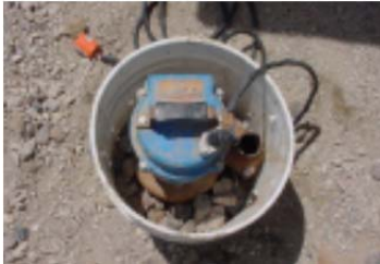
Sump pumps or suction lines can be contained within perforated 5-gallon buckets and surrounded with gravel to reduce the pumping of mud during dewatering operations.
