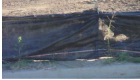
The lower edge of this silt fence is not anchored in a backfilled trench.
