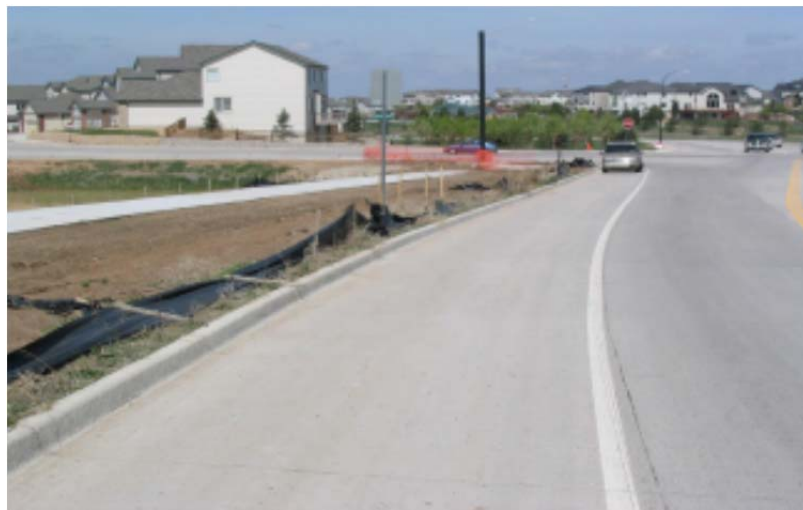
Maintenance procedures are not being followed on this site which may lead to additional costs from fines, sediment clean up and possible stop work orders.
