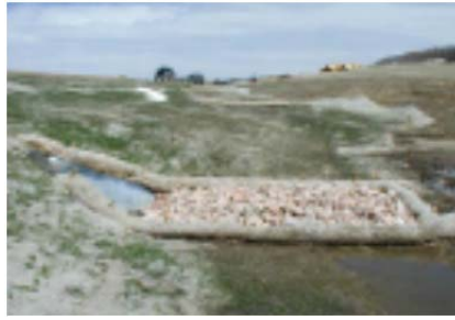
Although some sediment trapping would occur with this alternate arrangement, the standard detail shall be utilized.
