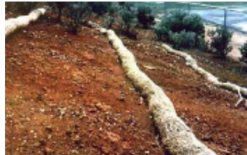
Sediment control logs may be used instead of silt fence on steep slopes.
