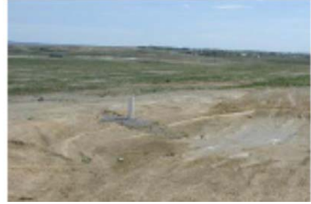
The sediment basin above is improperly installed due to:
