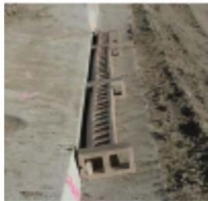
Temporary Inlet Protection. This interim configuration of blocks protects a street inlet prior to paving.
