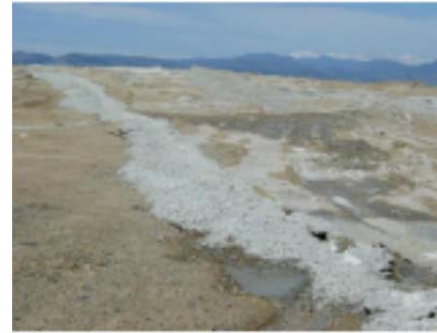
Extensive wasting of concrete on the construction site requires additional effort to clean up and can impair subsequent revegetation operations.
