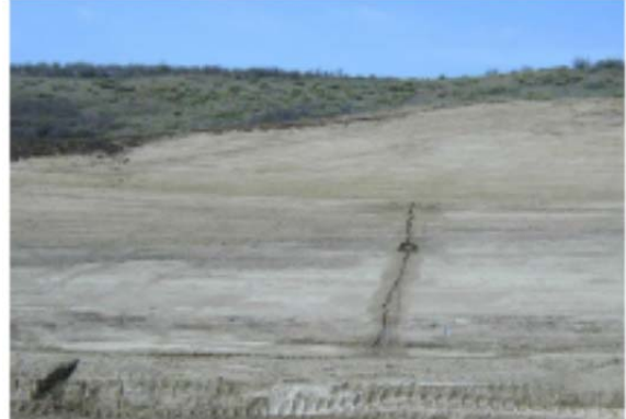
Surface roughening on this slope may have prevented this rill erosion.
