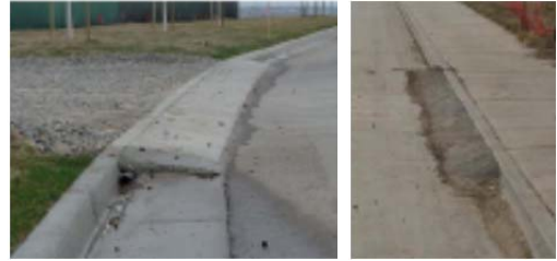
Curb ramps of earth, concrete, or lumber are not permitted in the curb section. Temporary ramps may be used.
