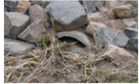
Without a reinforced rock berm for culvert protection, culverts fill with sediment.
