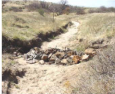
This check dam was not keyed in adequately to the channel bank, leading to its failure.
