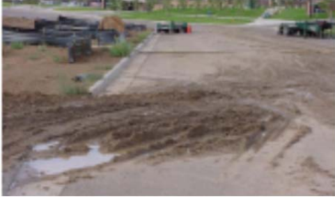
No vehicle tracking control means mud on streets and an immediate Stop Work Order.
