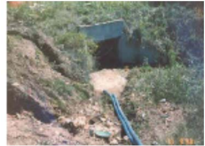
These discharge lines require a riprap pad and a settling trap.
