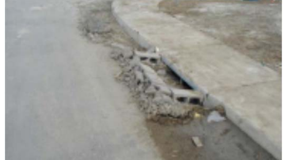
Tubular markers were not placed in front of this inlet protection installation, making it more susceptible to damage from snowplows and other vehicles. This installation is in need of immediate repair.
