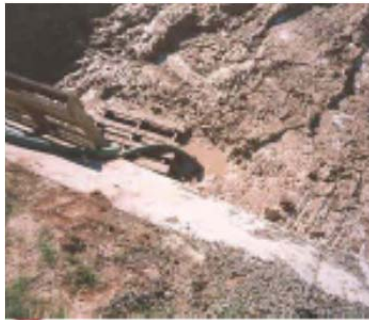
This suction line is not contained in gravel and is pumping excessive amounts of sediment.
