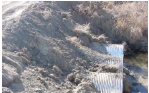
This temporary stream crossing is constructed of soil and is not acceptable.
