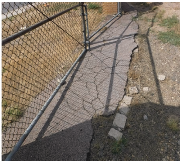
Blocked/Poorly Maintained Emergency Access
