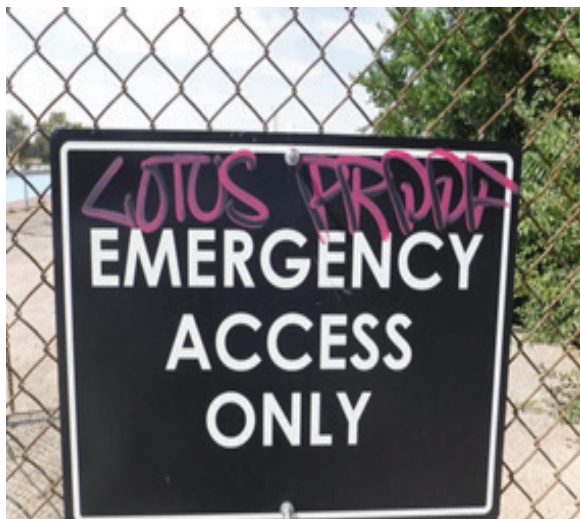
Deteriorated Signage via Graffiti
