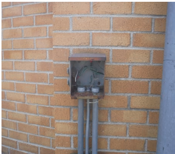
Unsafe/Exposed Electrical Wire
