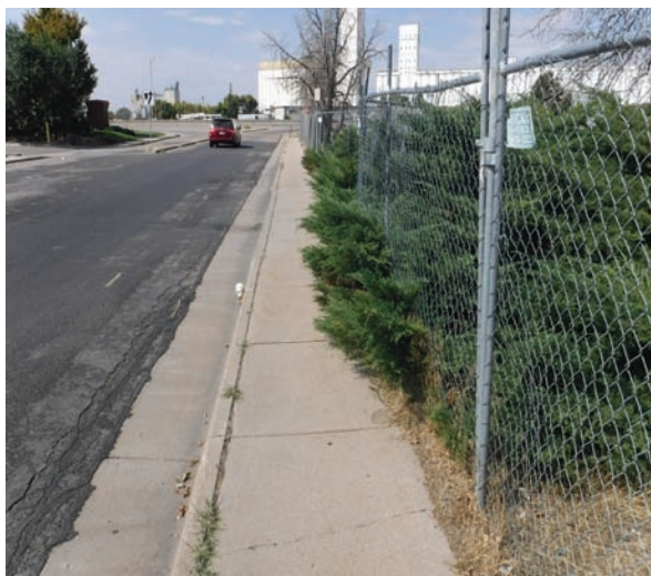
Pedestrian Barrier Resulting in Vehicle Conflict
