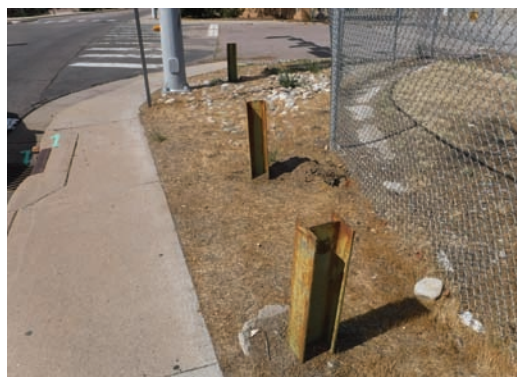
Deteriorated Accessory Structure
