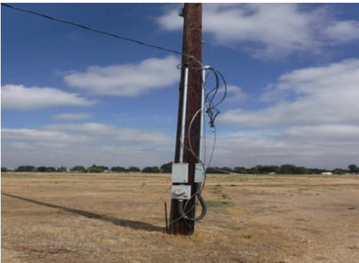
Deteriorated Electrical Pole
