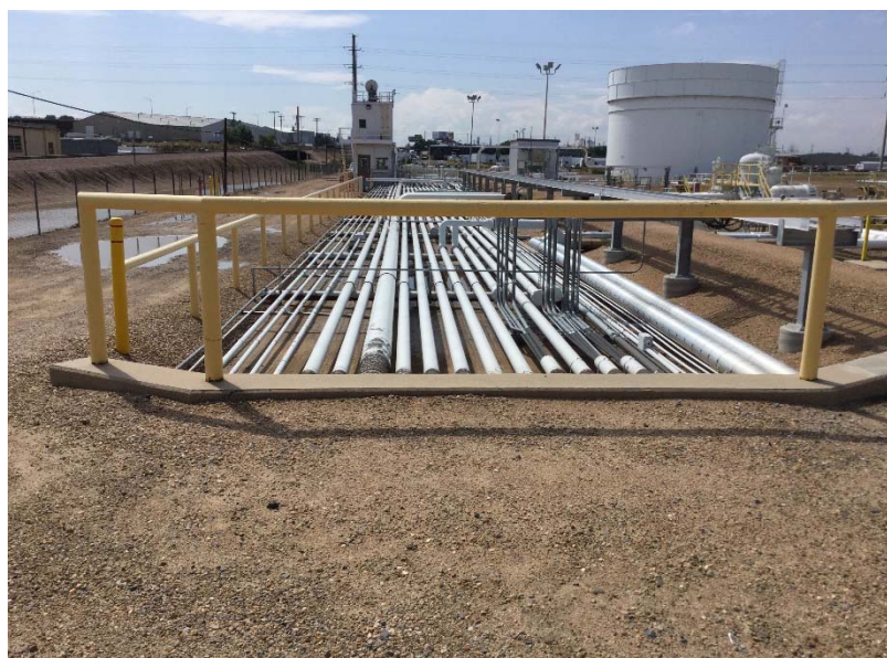
Equipment for Transfer of Product between Storage Tanks
