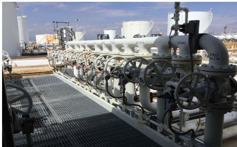
Equipment for Transfer of Product Via Off-site Pipelines
